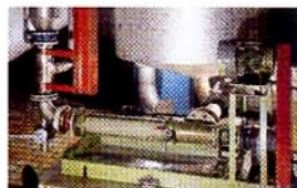
Crystallization Four seepex pumps BN 35-6L, product: high and low green molasses, flow: 4-25 m 3 /h / 18-110 usgpm, speed: 50-280 rpm, pressure: 2.7-3.2 bar / 40-45 psig, temperature: 70-85° C / 158-185°F, solids: 60-70% ds
