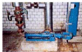
Crystallization seepex pump BN 17-6L, product: 'A' sugar run off, flow: 13 m 3 /h / 57 usgpm, speed: 265 rpm, pressure: 2.66 bar / 38 psig, temperature: 50° C / 122° F, viscosity: 200 mPas, SG: 1.4 kg/dm 3
