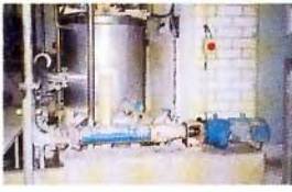
Application: metering additives/stock preparation. One seepex pump BN 52-6L with dry running protection TSE 120. Product: 50% pigment and 8% starch glue, flow rate: 40m 3 /h (175 gpm), speed: 265 rpm, pressure: 4 bar (60 psi), temperature: 24 - 50° C, Spec. gravity: 1.42
