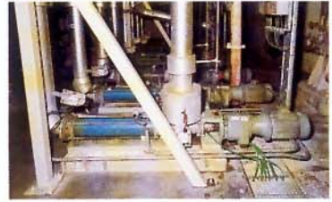
Application: coating kitchen. Eight seepex pumps BN 35-12 with dry running protection TSE 120 and flushing connection. Product: CMC or starch, flow rate: 15 or 25 m 3 /h (60/110 gpm), speed: 166 or 249 rpm, pressure: 12 bar (180 psi), temperature: 60 - 85° C, spec. gravity: 1.15, solids content: up to 30 - 35% wt, viscosity: 3500 - 5000 cps
