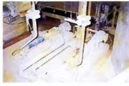
Application: metering additives/stock preparation. One seepex pump BN 5-6L with single-acting mechanical seal and dry running protection TSE 120. Product: CMC (carboxymethyl-cellulose), flow rate: 4.8 m 3 /h, speed: 350 rpm, pressure: 4 bar (60psi), temperature: 40° C, spec. gravity: 1.09
