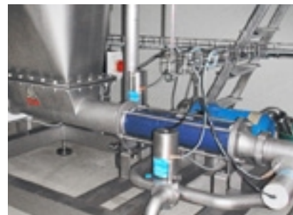
seepex pump BTCS 10-12, Product: tomato paste from containers, Temperature: 20°C (70°F), Pressure: 3 bar (45 psi), Viscosity: non flowable, Capacity: 0.5-1.3m 3 /h (2.2-5.72gpm)
