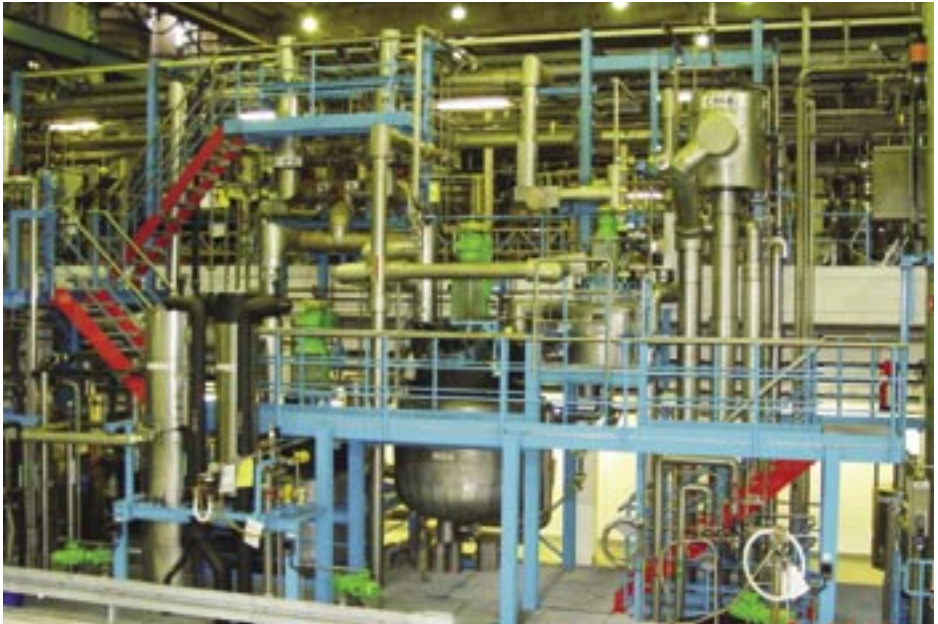
Picture 2: Distillery with zone 0 within the system and zone 1 in the surrounding building
