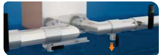
Stop the CIP machine. Drain the cleaning agent from the BPHE and CIP machine.
