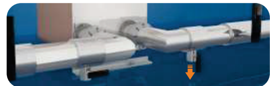
Stop the CIP machine. Drain the BPHE and CIP machine of cleaning agent.
